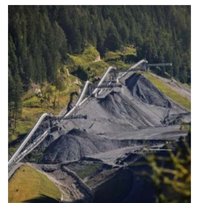
Conveyor belt system at the Brenner Base Tunnel (Padastertal landfill)
