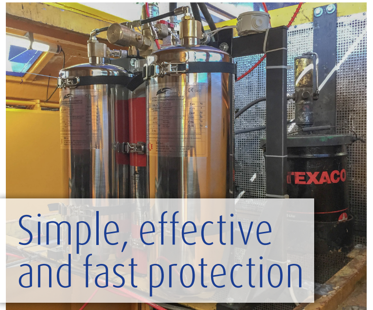
FALCON® fire extinguishing unit installed for engine protection
