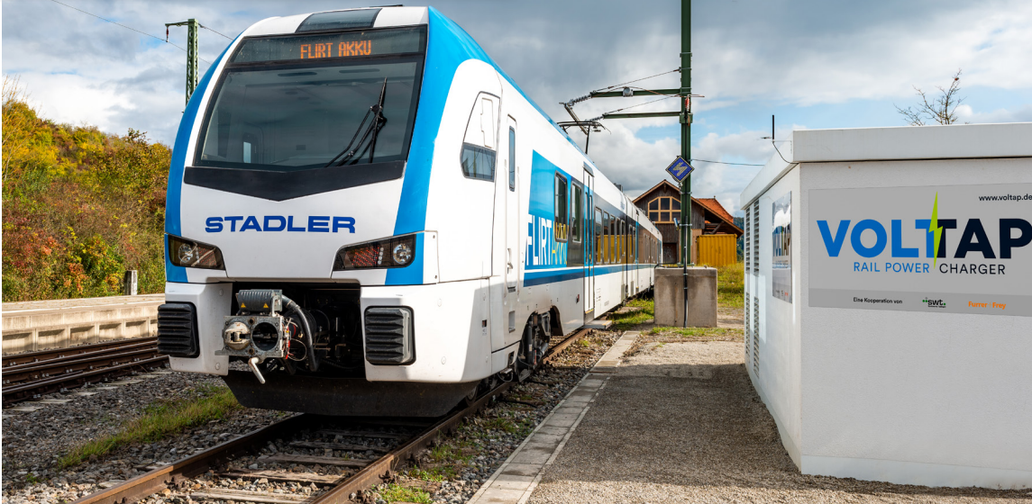
The VOLTAP rapid charging station consists of the transformer station (foreground) and an overhead line system (OLA) with charging masts and a charging rail. Photo: swt/Marquardt
